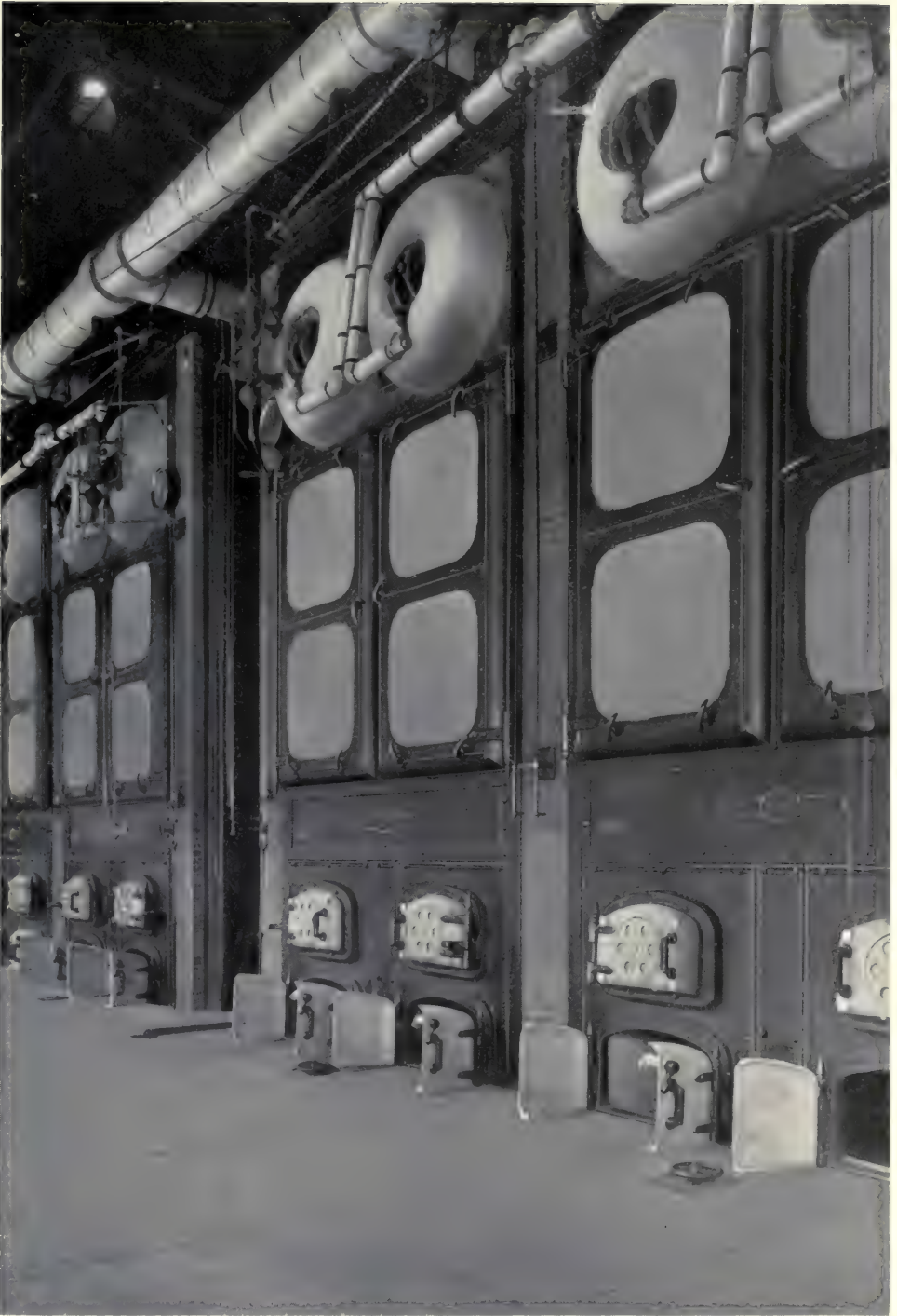
CARNEGIE NATURAL GAS CO., UNDERWOOD, W. VA. BABCOCK & WILCOX SUPERHEATERS INSTALLED IN 1600 HORSE POWER OF BABCOCK & WILCOX BOILERS
